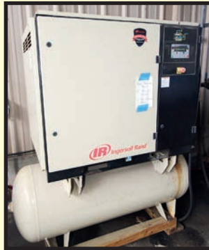
INGERSOLL RAND 30 HP AIR COMPRESSOR
