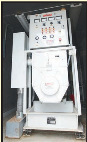
ALTURDYNE STAMFORD 134 KW 240 HP DIESEL GENERATOR
