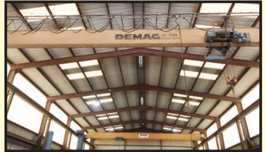
DEMAG 10 T. X 54' AND 7.5 T. X 54' CRANES
