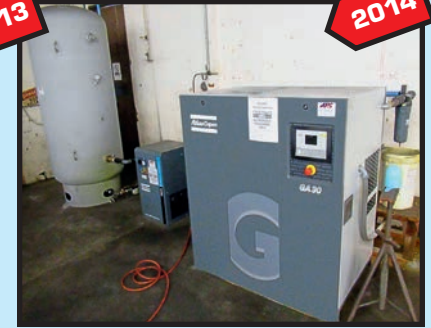
ATLAS COPCO 40 HP ROTARY SCREW AIR COMPRESSOR
