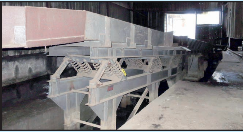
CARRIER APPROX. 60'L. INCLINED VIBRATORY PAN CONVEYOR
