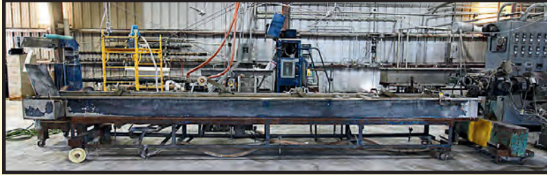
CUSTOM STAINLESS STEEL WATER BATH
