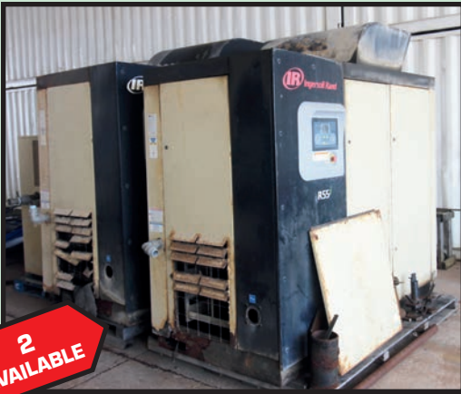
INGERSOLL RAND 55 HP ROTARY SCREW AIR COMPRESSOR
