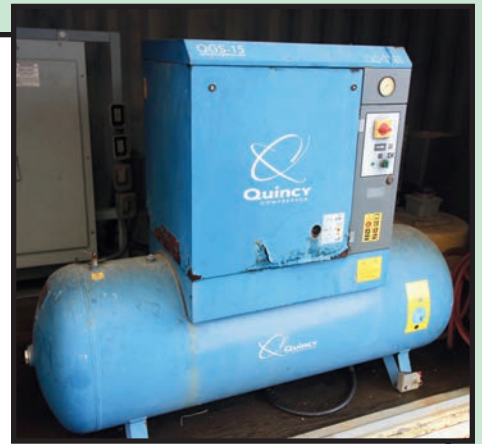
QUINCY 15 HP ROTARY SCREW AIR COMPRESSOR
