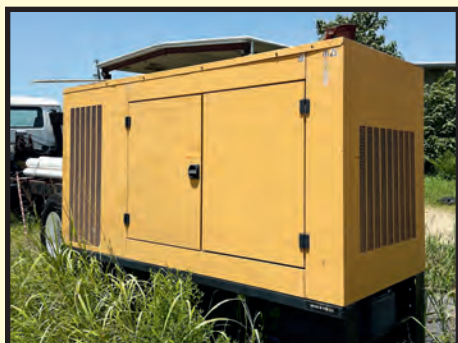
CATERPILLAR OLYMPIAN MDL. D150P1 GENERATOR
