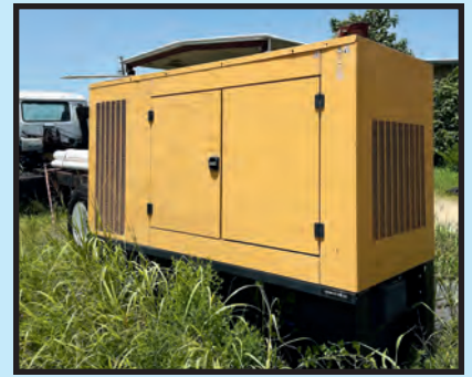
CATERPILLAR OLYMPIAN MDL. D150P1 GENERATOR
