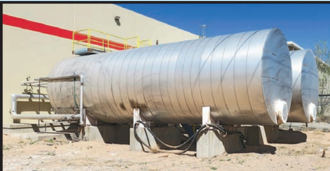
(2) LARGE INSULATED PROCESS TANKS
