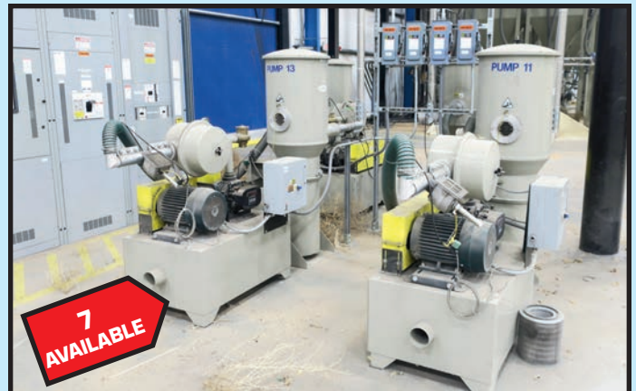
VIEW OF CONAIR 10 HP POSITIVE DISPLACEMENT PUMPS
