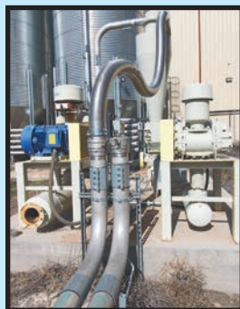
CONAIR DPDM RAILCAR UNLOADING SYSTEM
