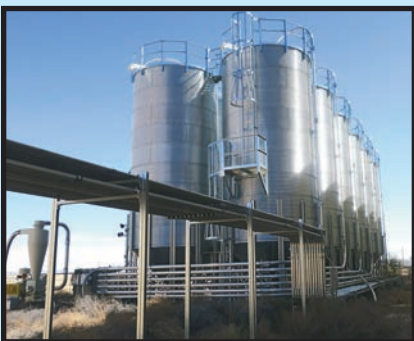
3,000 + FEET OF 2-1/2" O.D. ALUMINUM TRANSPORT PIPING
