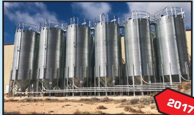
BULK UNLOADING AND STORAGE SYSTEM
