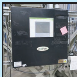
CONAIR CONTROL SYSTEM
