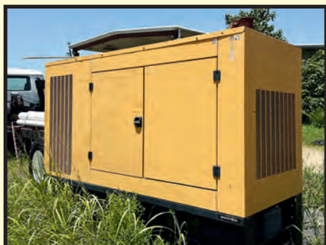
CATERPILLAR OLYMPIAN MDL D150P1 GENERATOR
