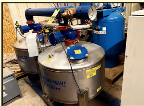
IRRIGATION-MART FILTRATION SYSTEM
