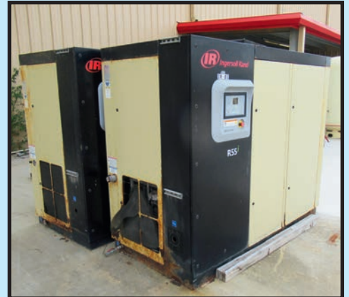
(2) INGERSOLL RAND 75 HP ROTARY SCREW AIR COMPRESSORS
