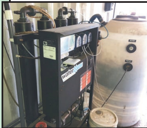
WATER MAZE COMPACT COAG WATER TREATMENT SYSTEM
