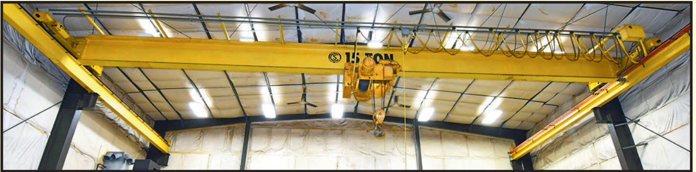
OVERHEAD CRANE SERVICE 15 T. CAP. X APPROX. 54' SPAN OVERHEAD BRIDGE CRANE
