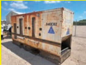
LOT 114: CAT SR4B GENERATOR powered by Cat 3304 diesel engine, equipped with 175KW, skid mounted. Not running.
