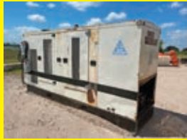
LOT 113: CAT SR4B GENERATOR SN:8CK00615 powered by Cat 3304 diesel engine, equipped with 175KW, skid mounted. Not running.
