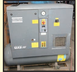
ATLAS COPCO GX5FF AIR COMPRESSOR
