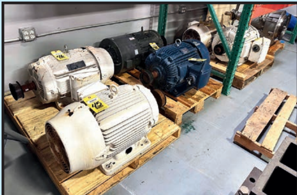
SAMPLE VIEW OF ELECTRIC MOTORS
